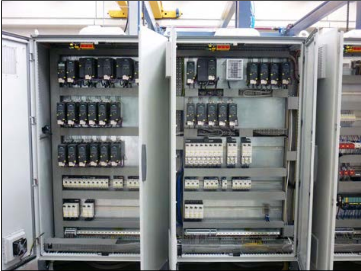
Main electric cabinet
